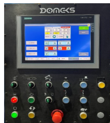
Fig. 4. Main Control Panel
